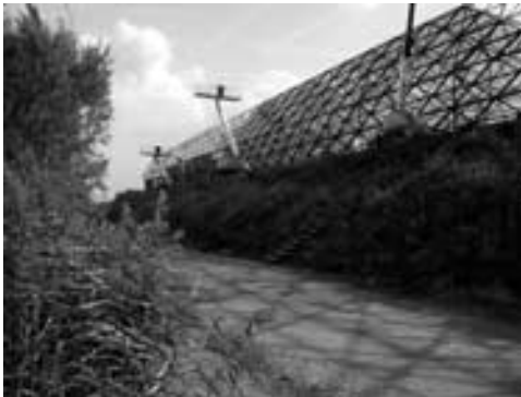
Fig 5C: Acoustic Barrier, ONL [Oosterhuis_Lénard] 2004, Building site progress, 15 September 2004, the Cockpit will connect to the left end
